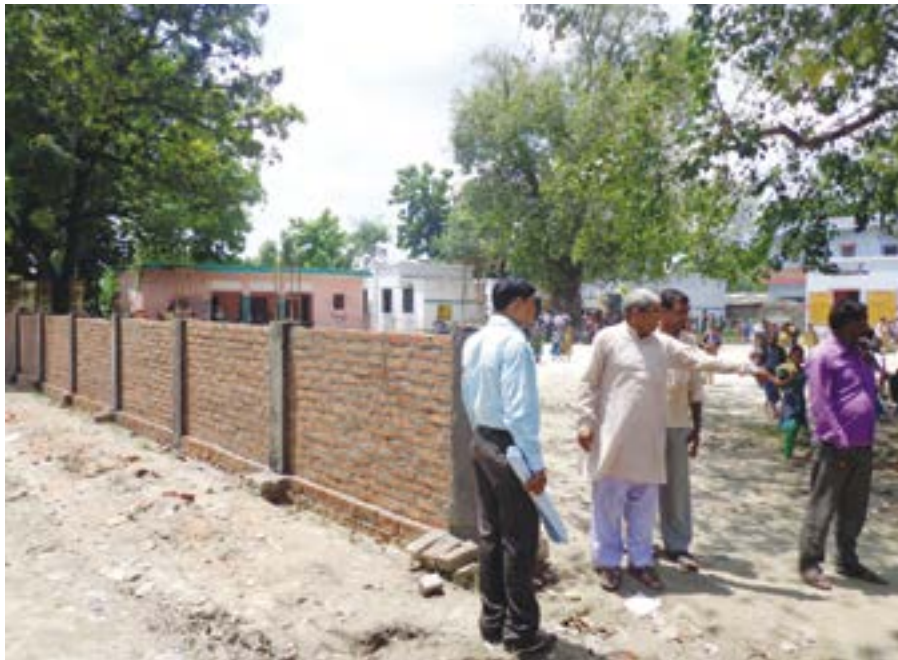
School Management Committee members monitoring the construction of a boundary wall at Mansa Chapar, Siswa block Mahrajanj district
